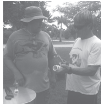
Glen Gareau and Joe Evans installing the new water fountain at the duck pond.
